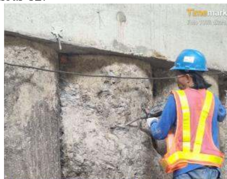
Gambar 12 Pembobokan Major Bulging
